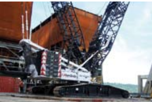
AmQuip's newest LR1400 is working for Bechtel in Trimble County, KY. The machine is configured with full superlift, making lifts in excess of 390,000 pounds
