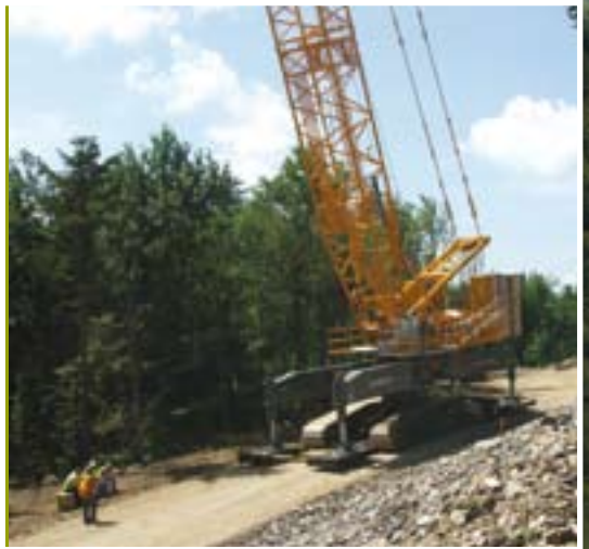
Northwest Cranes' Liebherr LR1400/2-W Narrow Track has been ideal for the narrow roadways at a wind farm in New Hampshire. The narrow track is also less damaging to the terrain
